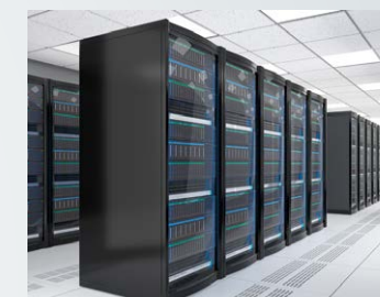
Data centers that support high-capacity communication
