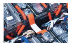
Connection resistance of battery busbars
