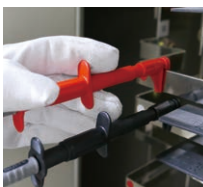
For clamping around the target busbar
